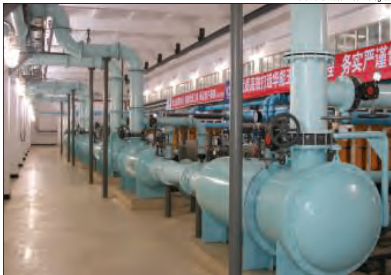
FIGURE 2. This photo shows an installation of an RO high-pressure pump and the energy recovery devices (in the background)
