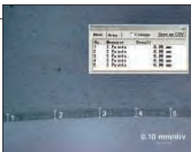
FIGURE 5. After 17 years of continuous contact with 35 wt.% hydrogen peroxide (25°C), only 60 µm of corrosion attack is measured with PVC-U piping components. Such minor traces of corrosion do not influence the function or safety of the system at all
