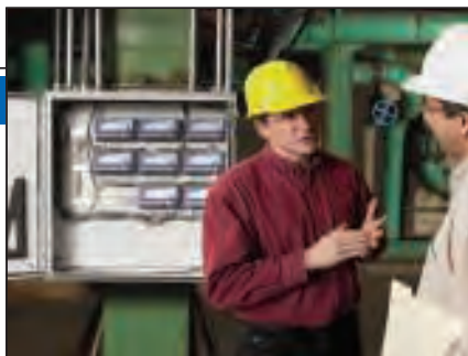
FIGURE 5. High density transmitters, such as these, can accept up to eight thermocouple or RTD inputs each, thus replacing many individual wire runs in applications such as columns and reactors
