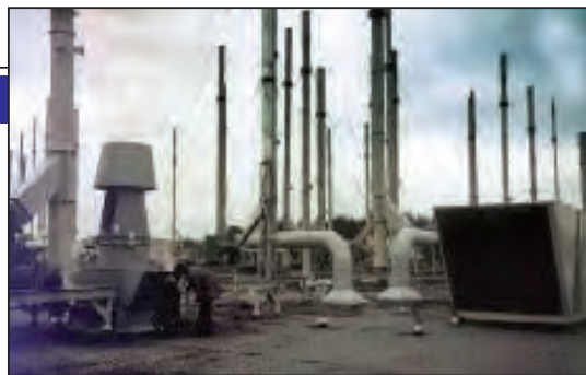
FIGURE 2. A difference between exhaust system types is the height of rooftop stacks, a characteristic with value in accommodating space and weight restrictions
