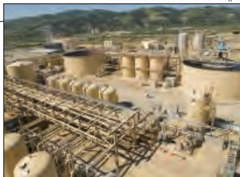
FIGURE 1. Pictured is a Chevron facility in San Ardo, Calif., where Veolia's OPUS system has been operating
