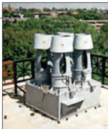
FIGURE 1. Roofline aesthetics are among a host of considerations when selecting a fume-hood exhaust system for a laboratory facility
